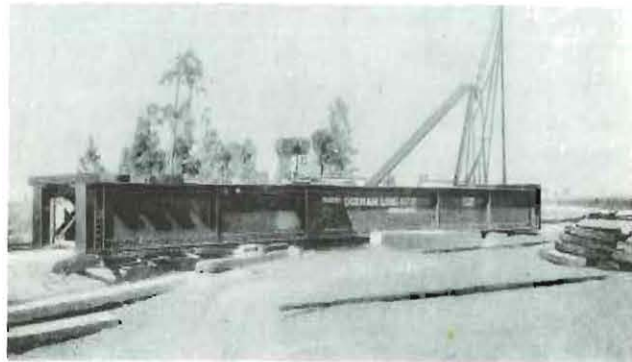
ONE OF THE NEW SPANS SHOWING RIVETING, PAINTING AND FIXING OF SLEEPERS IN PROGRESS AT THE SAME TIME ON DIFFERENT PARTS OF THE GIRDERS
