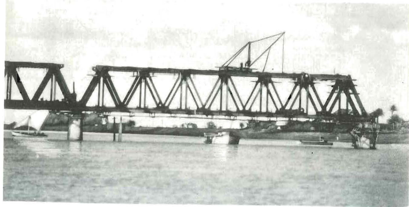
SPANS Nos. 7 & 8. ERECTION TIES REMOVED, BUT GUSSET PLATES NOT YET CUT AWAY
