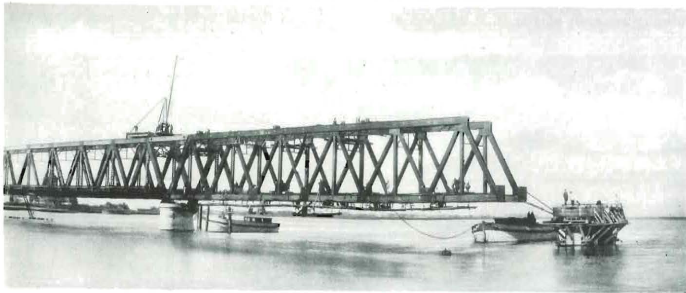
PHOTOGRAPH TAKEN AS THE BRIDGE APPROACHED COMPLETION, SHOWING OVERHUNG SPAN REACHING ALMOST TO THE NEXT PIER, THE TEMPORARY TOP CHORD TIES CAN PLAINLY BE SEEN
