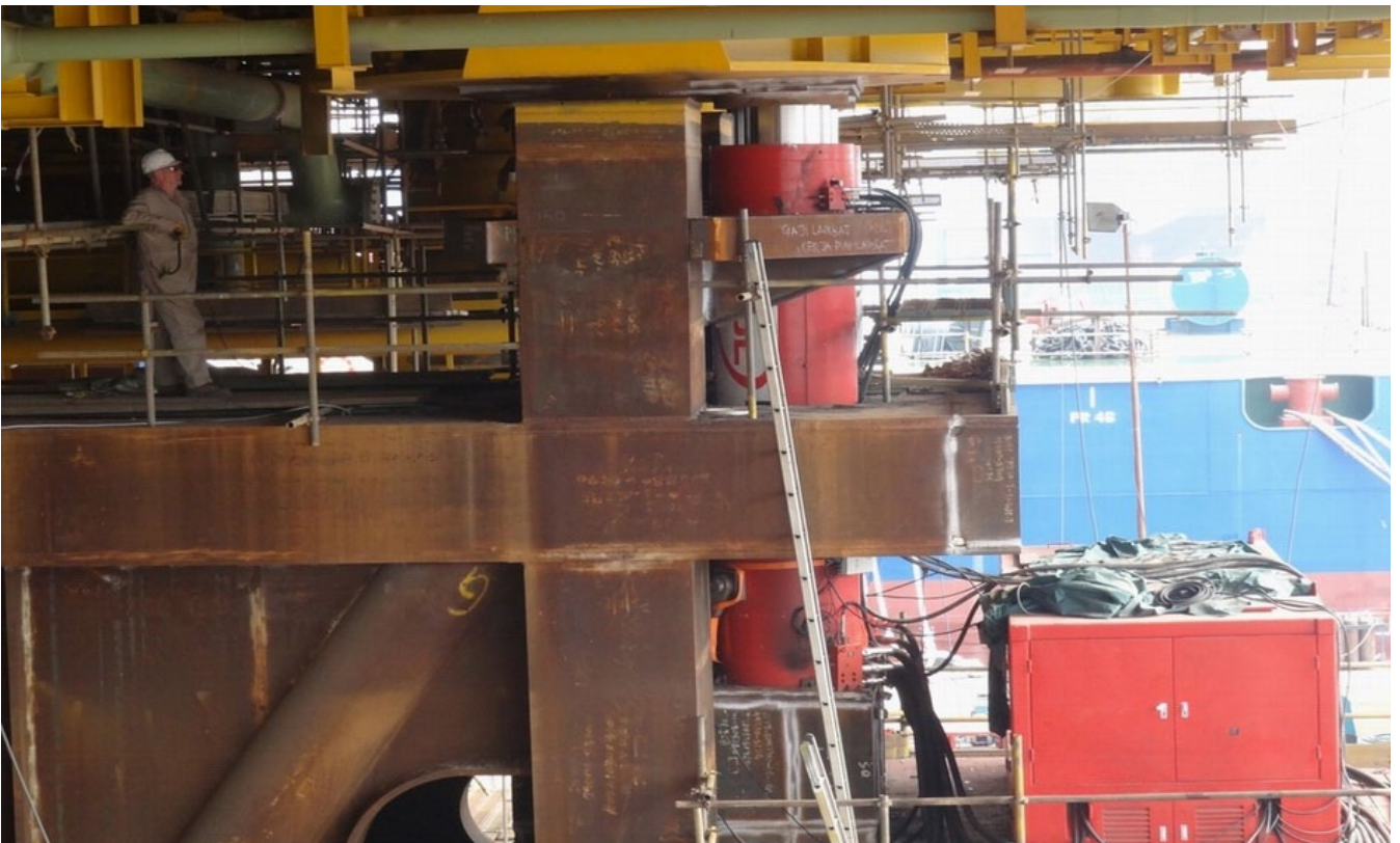
16 No 1250 MT jacks with 2000mm stroke, being used for onshore weighing of a topside using hydraulic pressures for a load measurement accuracy of 1% after correction for seal friction.
